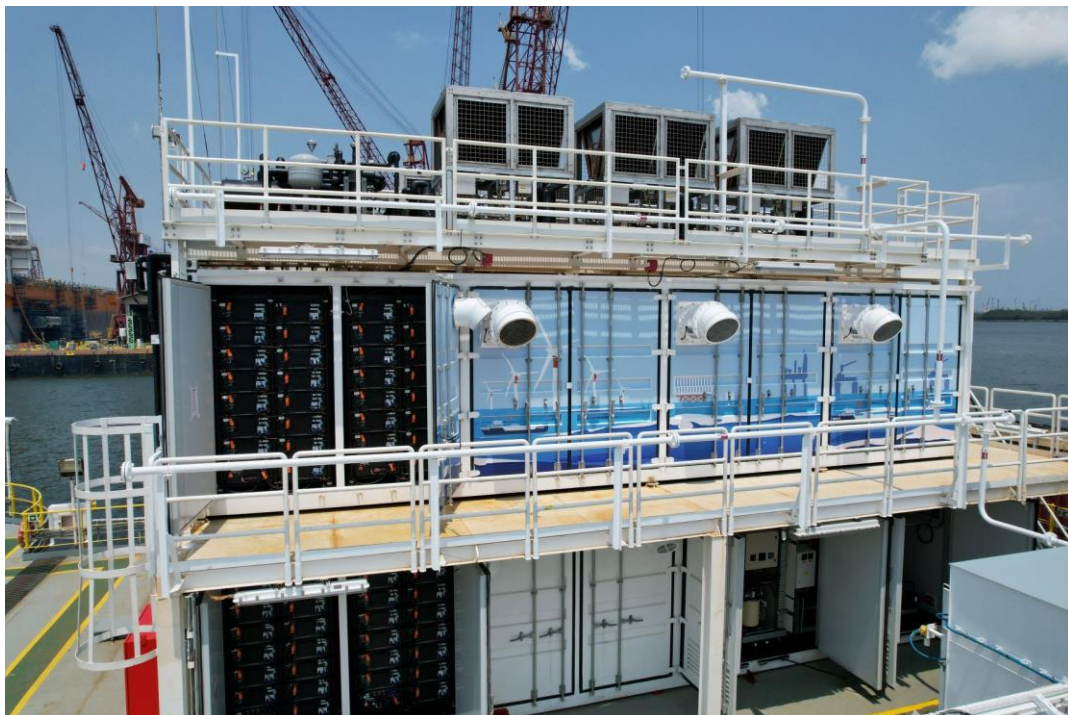
Photo of Southeast Asia's first floating and stacked Energy Storage System, with maximum storage capacity of 7.5 megawatt hour (MWh) to power over 600 four-room HDB households in a single discharge. (Photo credit: Seatrium Ltd)
