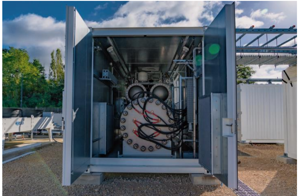
Caption: Electrolyser Photo credit: EDF HQ Singapore Pte Ltd
