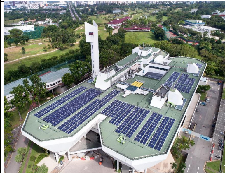
Aerial view of the SolarRoof installation on Jurong Town Hall.
