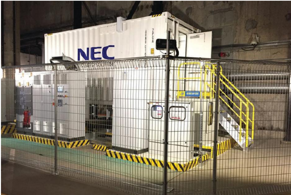
Figure 9: Self-Regulating Integrated Electricity-Cooling Networks (“IE-CN”) at the Marina Bay district cooling system [Courtesy of Singapore District Cooling Pte Ltd]
