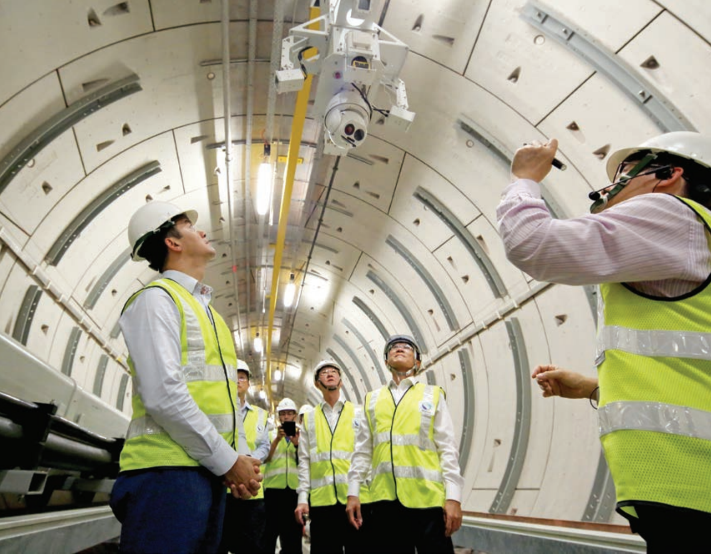
^ Automatic inspection vehicles and smart sensors are used to monitor and detect any abnormalities in the electricity cable tunnels.
