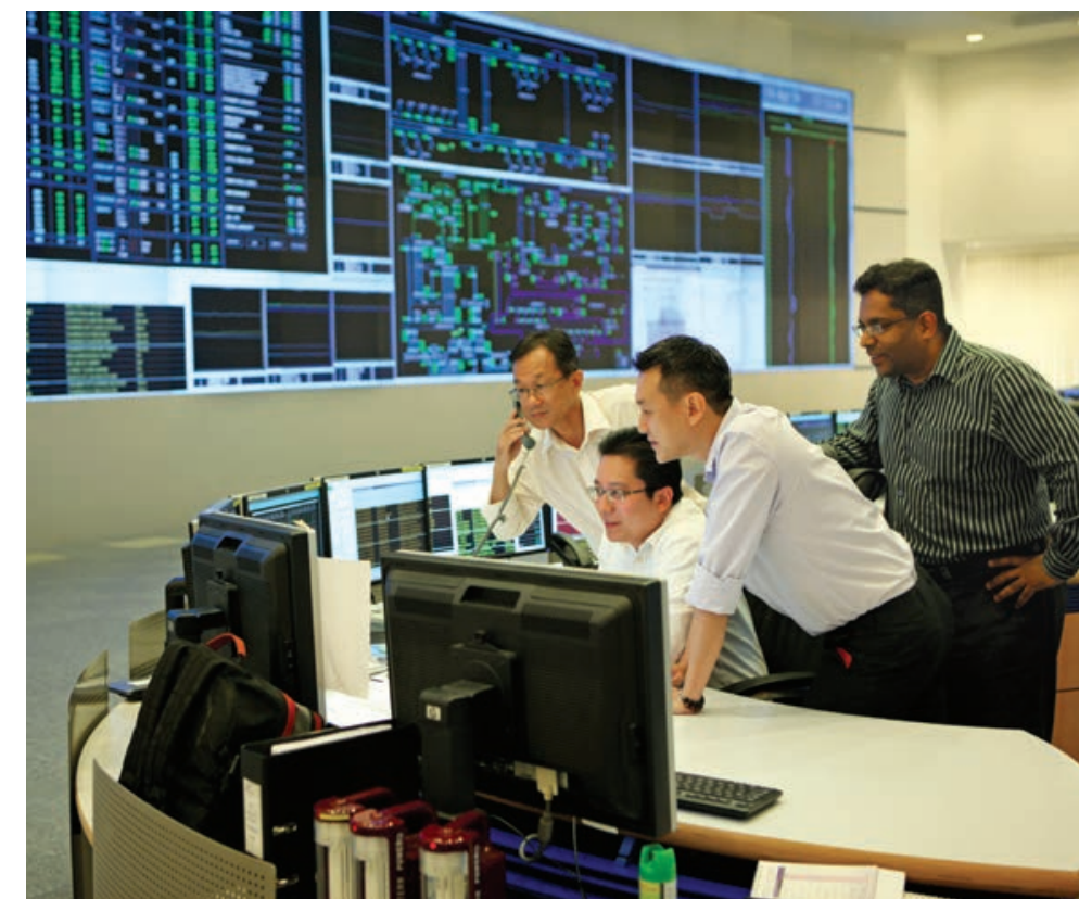
↗ EMA officers manning the Power System Control Centre, the nerve centre of Singapore's electricity generation and transmission system.
