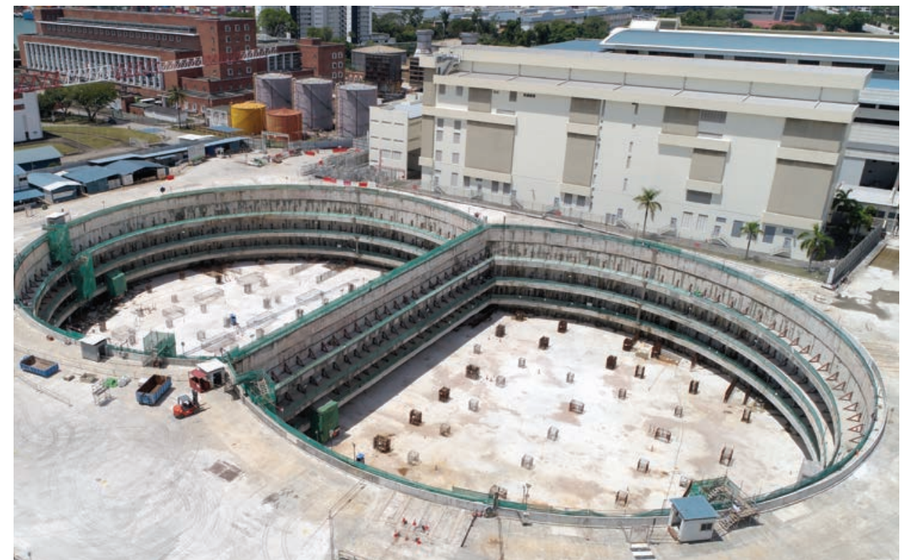
^ Site of Singapore's first large-scale underground substation at Labrador, which is scheduled for completion in 2024.
