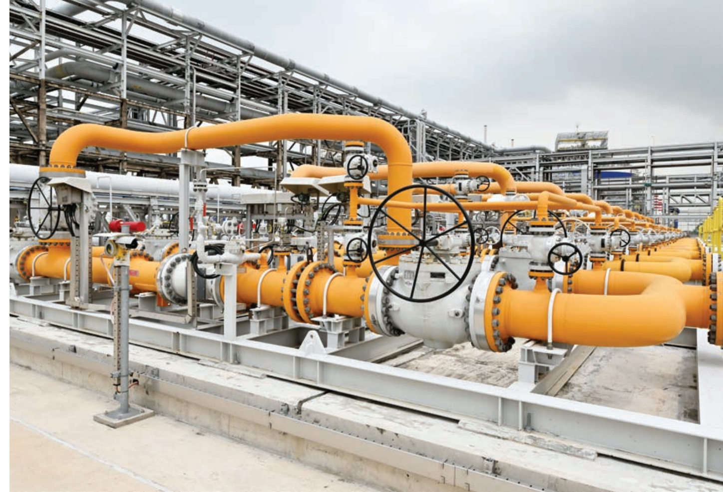
^ Natural gas is a reliable source for power generation.
