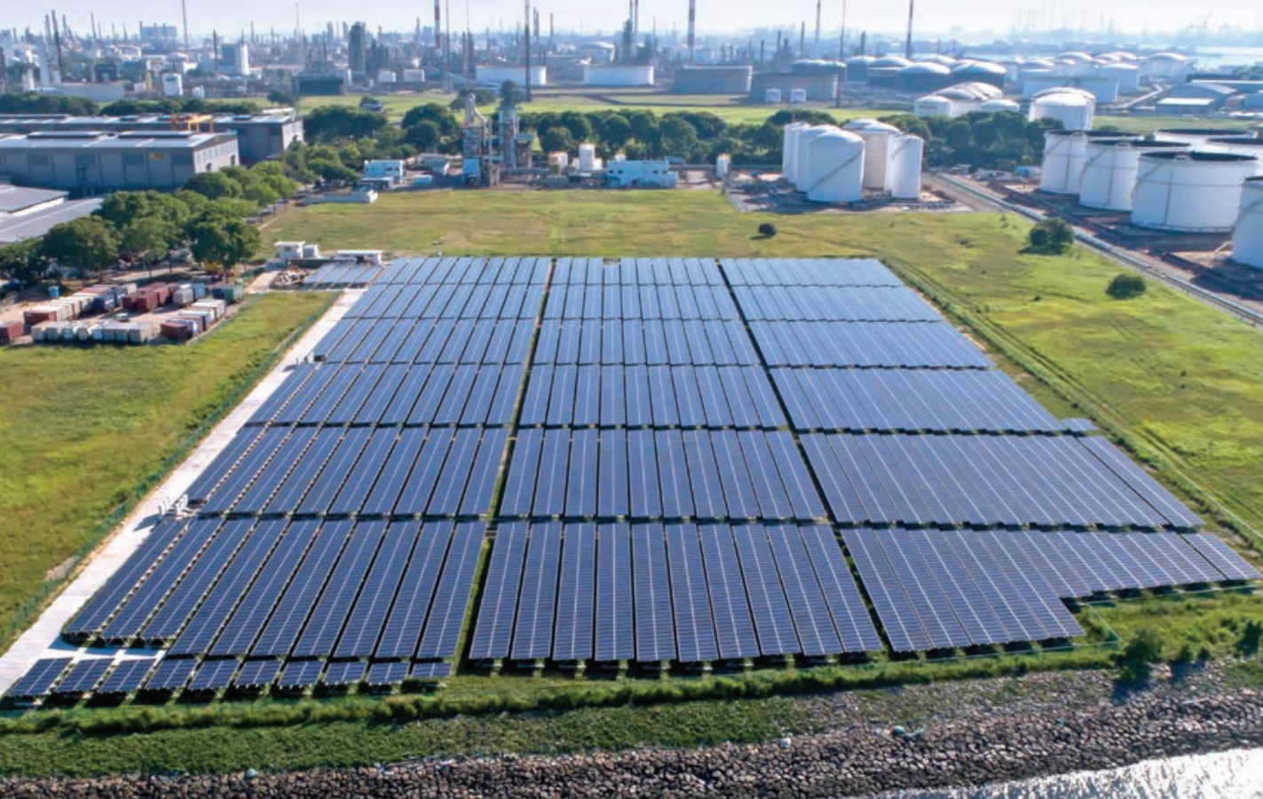
^ Aerial view of the SolarLand installation on Jurong Island. The system is modular and flexible, allowing JTC to maximise temporary vacant land and redeploy the panels when the land is needed.
