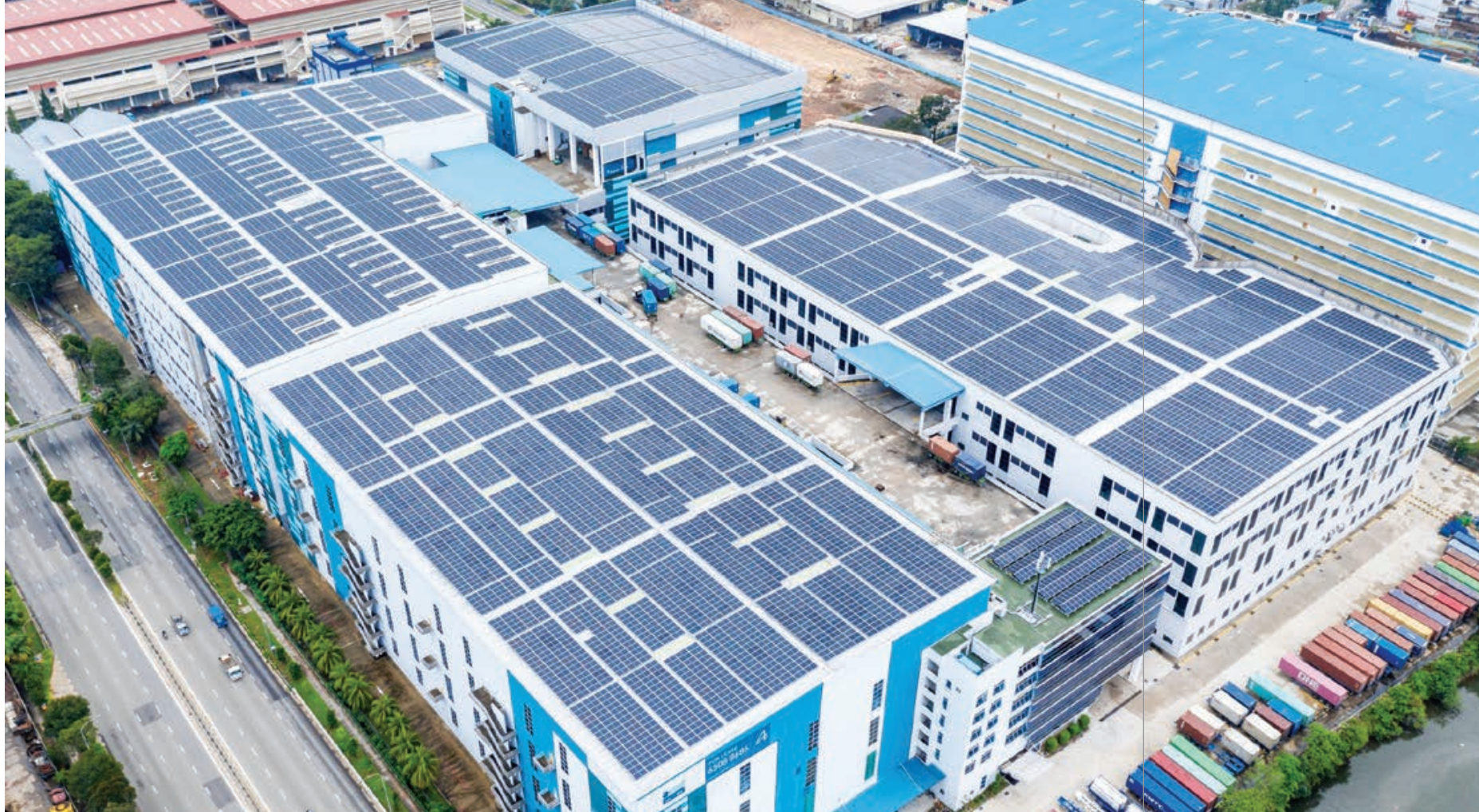
^ The rooftop installation at Ascendas Real Estate Investment Trust-owned facility at 40 Penjuru Lane, which enabled Singapore to cross its 2020 solar deployment target of 350 megawatt-peak (MWp) in the first quarter of that year.
