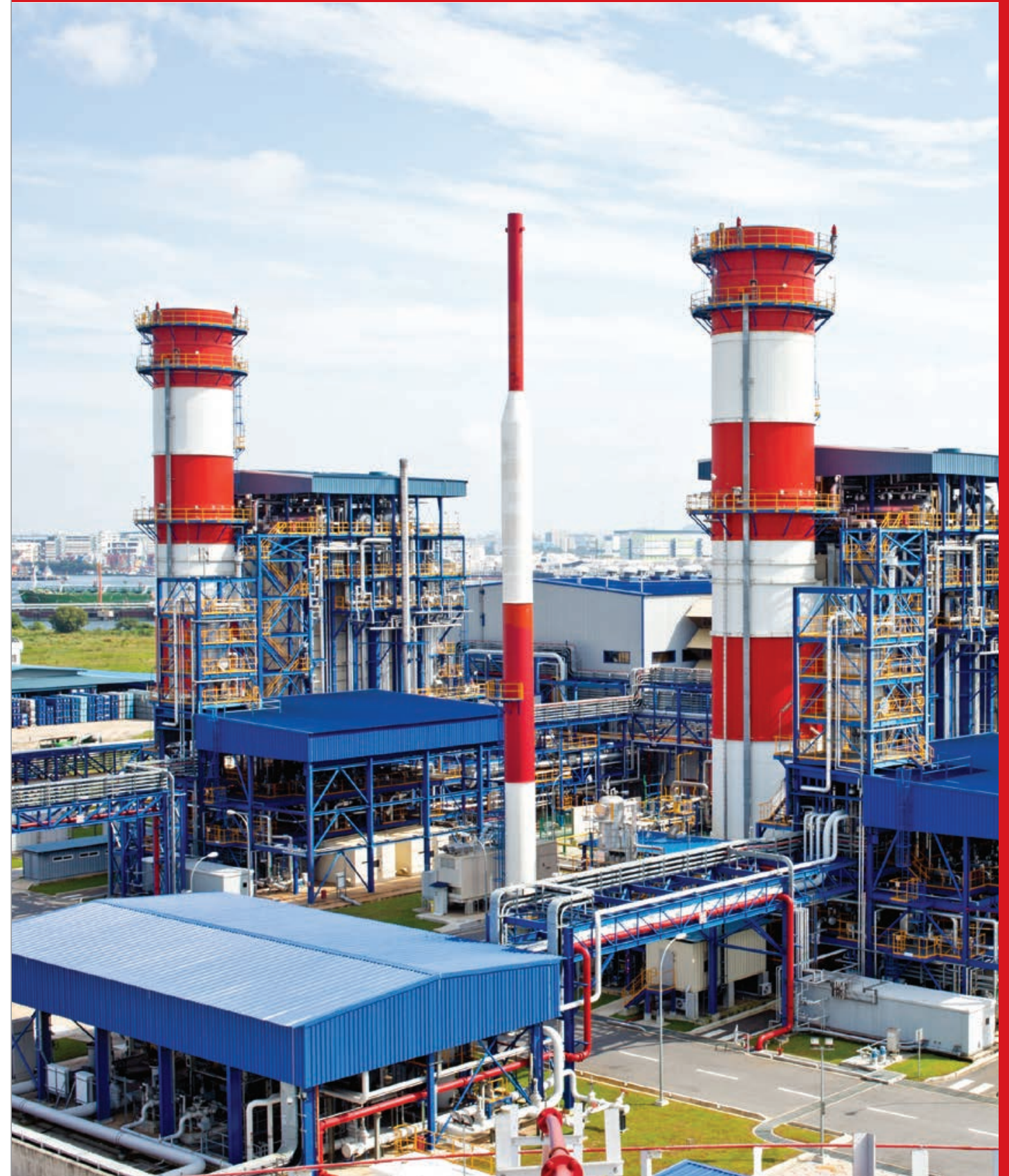
^ The 800 megawatt Combined Cycle Gas Turbine power plant by PacificLight Power Pte Ltd.
